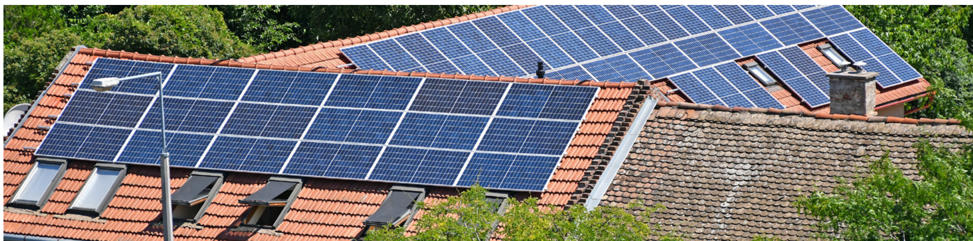
Solar panels on the top of a building, Hungary
